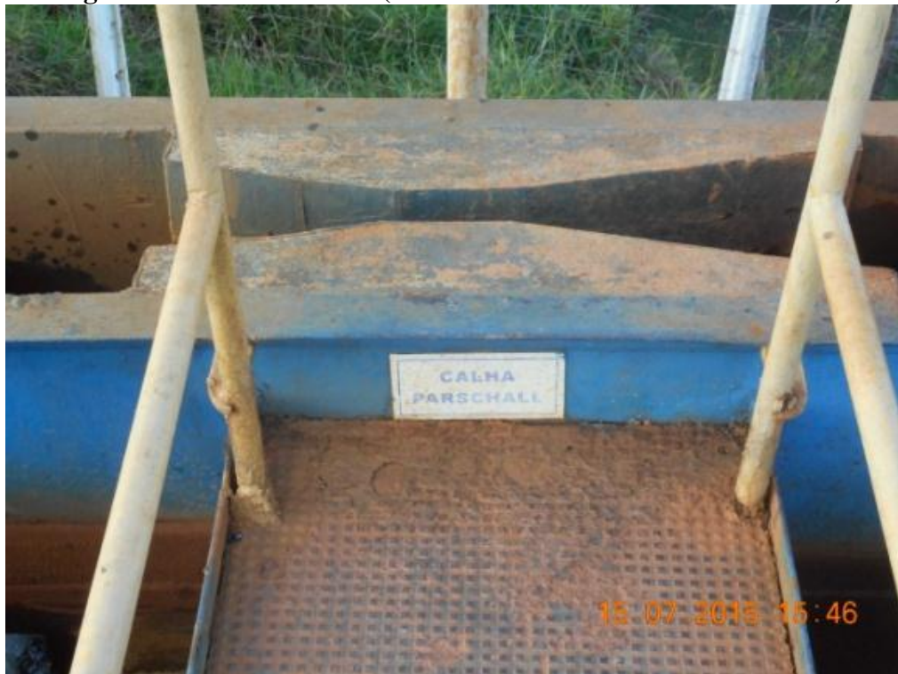
Figura 33: Calha Parshall (Local: S 18°57'54.6'' W 043°15'06.5'')
